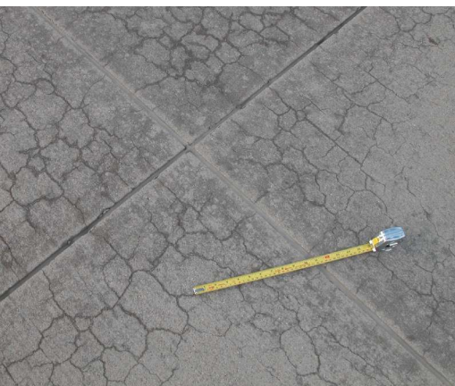
Photograph of map cracking on concrete pavement affected by alkali-silica reaction. All Photos and Figures: Dr. David Rothstein.
