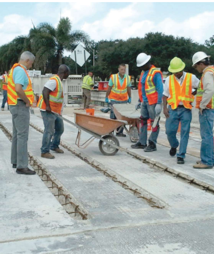
Ultra-high-performance concrete repair of connections between precast, prestressed concrete voided-slab beams in Florida. Photo: Florida Department of Transportation.
