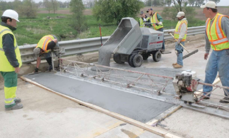
The first installation in the United States of an ultra-high-performance concrete bridge deck overlay was in Iowa. Photo: Federal Highway Administration.
