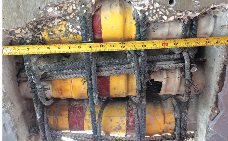
Ultra-high-performance concrete was used for the repair of a midspan spliced U-girder closure pour. Photo: SEMA Construction Inc.
