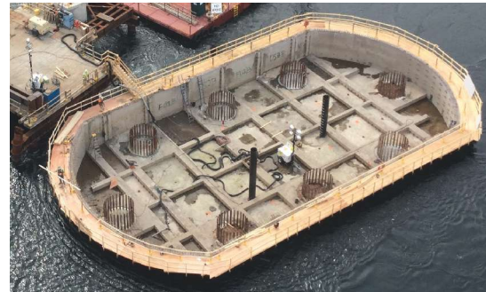
The dewatered tub with the drilled shafts visible. The work platform has been attached to the top of the tub. Photo: Cianbro.
