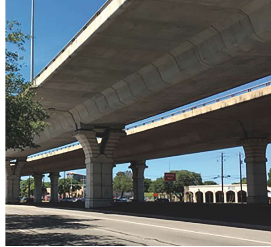
Service IV load combination was used to design the precast concrete segmental substructures for the U.S. Route 183 elevated viaduct in Austin, Tex. Photo: Dr. Oguzhan Bayrak.
