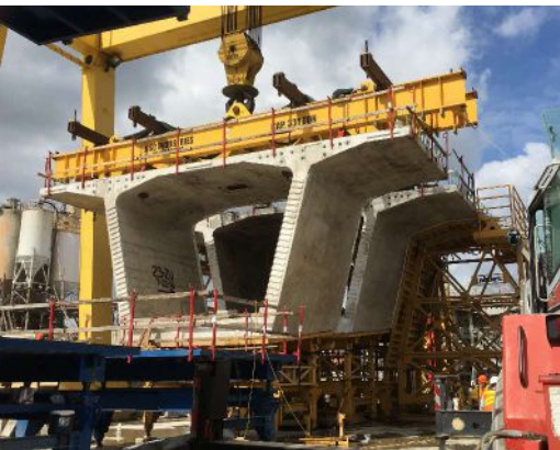
Precast concrete segments were match-cast under controlled conditions at an off-site precast concrete facility, which resulted in high-quality, durable components.
