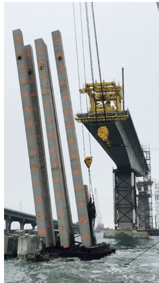
Creative pile templates were used to control the geometry during installation of battered 36-in.-square piles that were at least 130 ft long.
