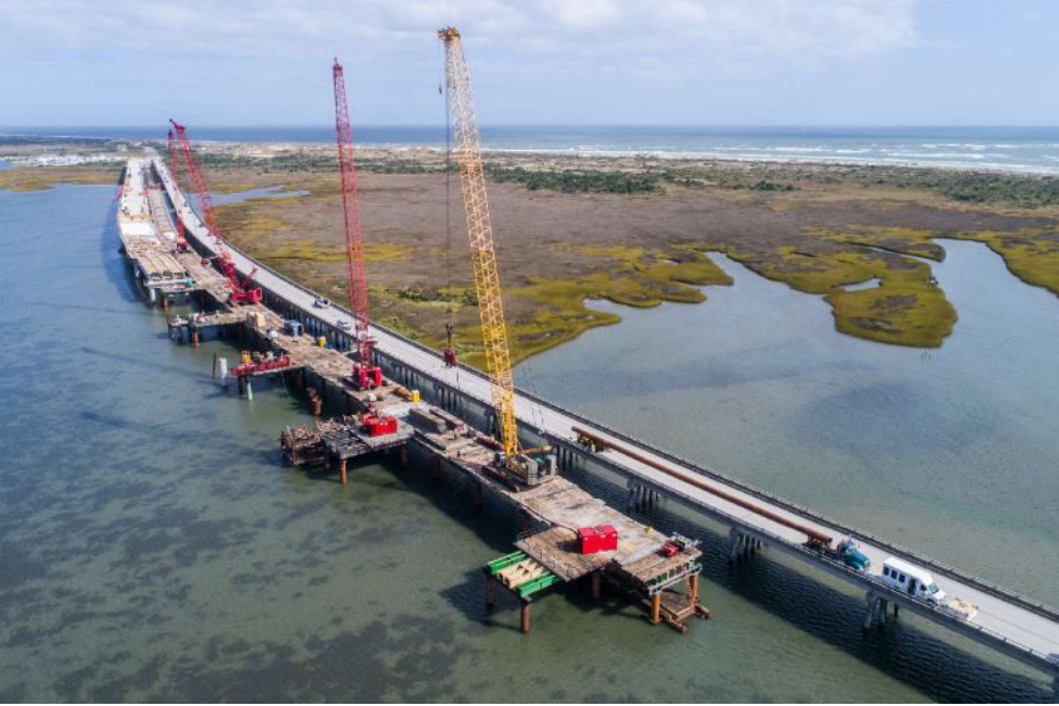
An innovative “leapfrog” approach to work-trestle construction for the north approach spans reduced the project’s temporary environmental impact associated with shading of seagrass beds.
