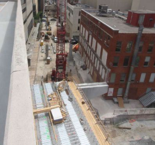
Several prestressed concrete girders have been placed for the span in the foreground. Because of the confined site, the crane had to back out after all girders were set for a span so the cap for the next span could be constructed.
