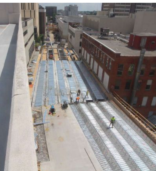
Prestressed concrete girders have been erected and forms set for placement of the deck.
