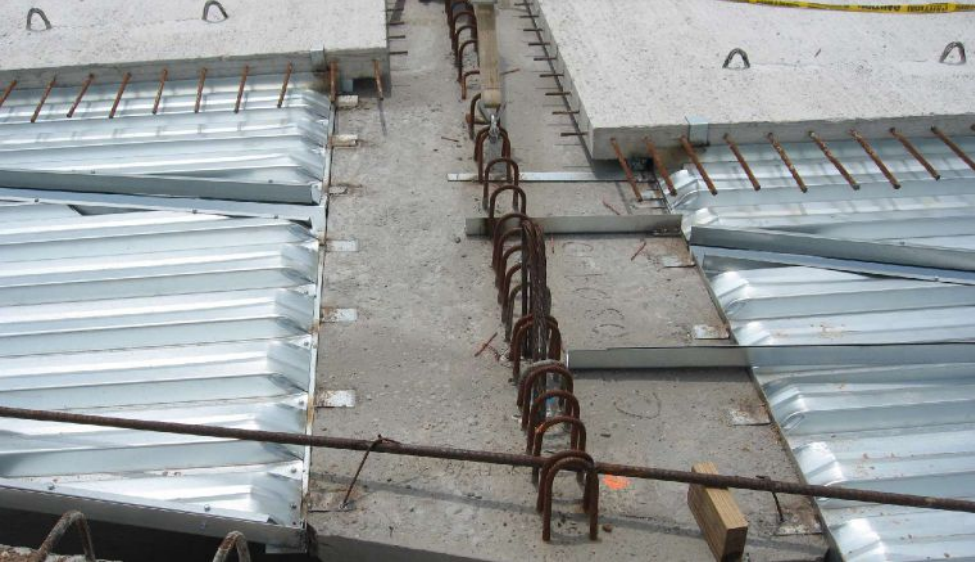
Old detail at the girder end showing the stay-in-place metal formwork on each side of the girder. Photo: John Holt.
