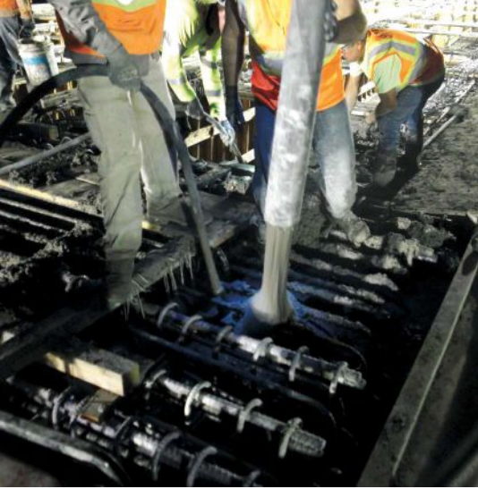
Placing lightweight concrete for bent caps by pumping. Because of the high cementitious materials content, active (cooling tubes) and passive measures were used to control the concrete temperature to avoid thermal cracking and the potential for later cracking caused by delayed ettringite formation.
