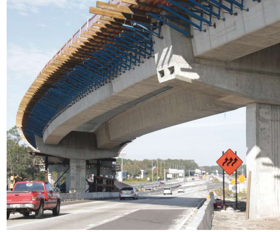
Curved precast concrete U-girder span over Interstate 95 during U-girder construction. The girders are supported with integral cast-in-place concrete diaphragms made composite with precast concrete pier caps. Photo: Seidler Productions.
