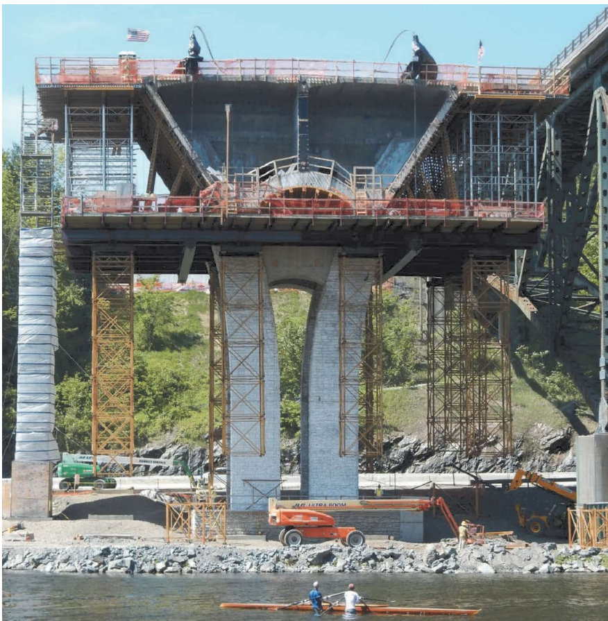
Construction of Pier Table 1. Pier 1 soared 70 ft in the air while vehicular traffic was maintained on Route 30 and river remained open for recreational boating.
