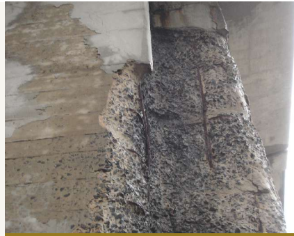
Close-up view of same pier showing loss of concrete cover at pier corner. Photo: WJE.
