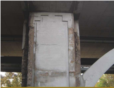
Concrete deterioration and reinforcement corrosion below deck expansion joints. Photo: WJE.
