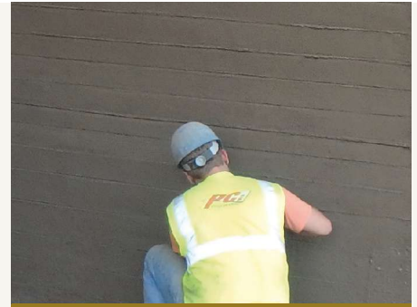
Applying board-form finish to dry-method shotcrete repair on the underside of an arch rib. Photo: HNTB.
