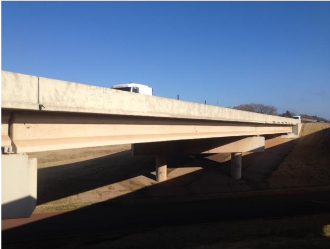
Figure 1. I-35 Southbound over Rollercoaster Road and Pine. Logan Co., OK. The photograph highlights spans 2 and 3 which were made with AASHTO Type IV girders. Span 2 spans 103.43 ft. with girder spacings at 8.20 ft. The bridge was built in 1998 with straight strand patterns that replaced draped strand designs. Strand patterns included fully tensioned “top strands” to mitigate the number and length of debonded strands. This bridge was the first of 700 bridges built in Oklahoma that incorporate designs with straight strand patterns and fully tensioned top strands, and limited debonding where required to control end zone stresses. The practice continues through today. Photo taken by Bruce W. Russell, 2014.
