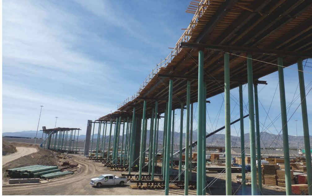
Falsework in place for frame 2. The maximum falsework height was 58 ft. Photo: Nevada Department of Transportation.
