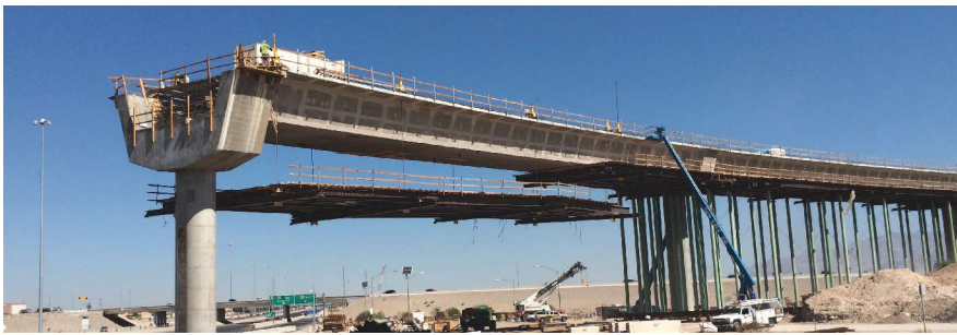
Falsework of frame 2 being lowered after completion. Photo: Nevada Department of Transportation.
