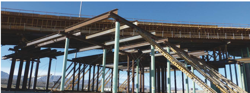
Frame 3 tunnel bent over U.S. Route 95 with bracing. Photo: Nevada Department of Transportation.
