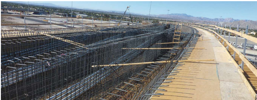
Concrete box girder with reinforcement and post-tensioning ducts in place for soffit and webs. Photo: Nevada Department of Transportation.
