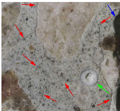
Figure 2. Reflected light photomicrograph of the polished surface of a core from a concrete structure with delayed ettringite formation. Arrows indicate microcracks that are filled with a clear, gel-like material (red), a void filled with ettringite (green), and the outer surface of the core (blue).
