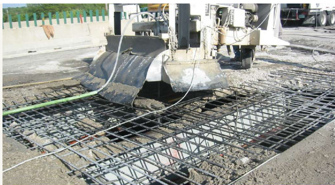
Full-depth deck concrete removal. Note the very clean condition of the reinforcement.
