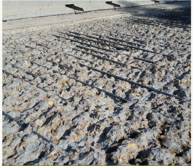
Fast-track hydrodemolition surface showing selective removal of deteriorated concrete areas. The process provides a clean, etched, and bondable surface ready for an overlay.
