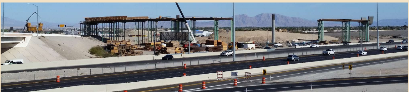
Progress photo of placement of falsework for frame 2. Photo: Nevada Department of Transportation.
