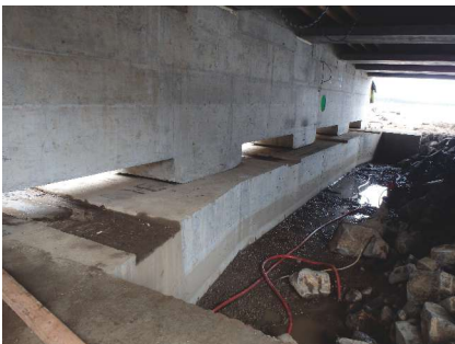
Lochner used nonproprietary equipment to slide into place the Lardo Bridge, carrying State Highway 55 over the North Fork of the Payette River in McCall, Idaho.
