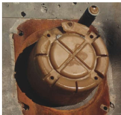
Flexible filler encapsulation of post-tensioning wedge plate (grout cap removed). Photo: Florida Department of Transportation.
