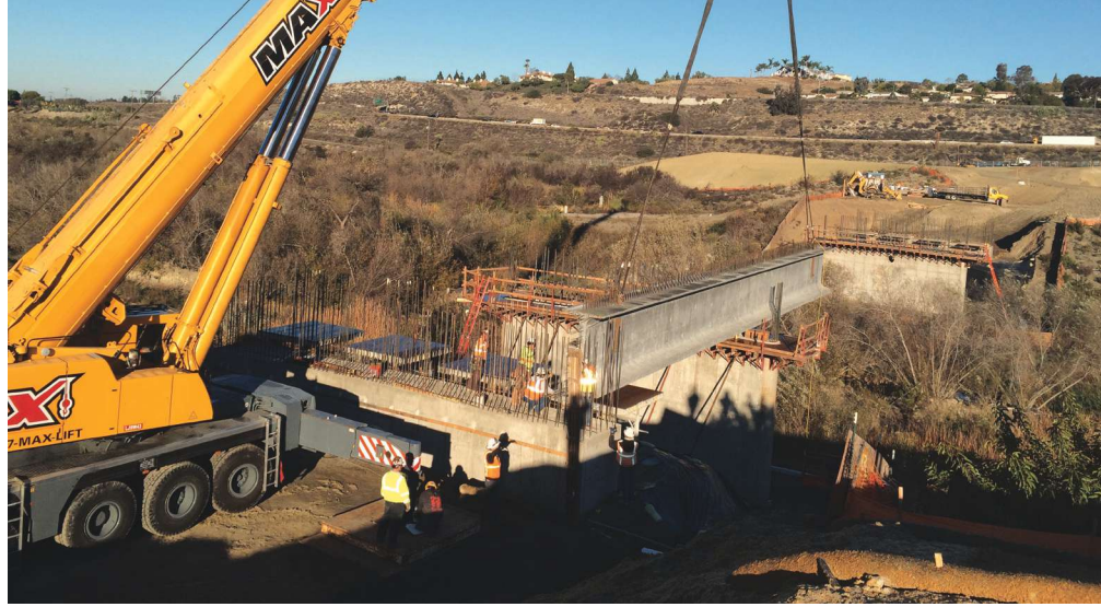
Phase 1 construction included placement of end girder on shoring towers at the abutments and timber blocks on the piers. The end girders cantilever 29 ft past the pier and extend over the environmentally sensitive area.
