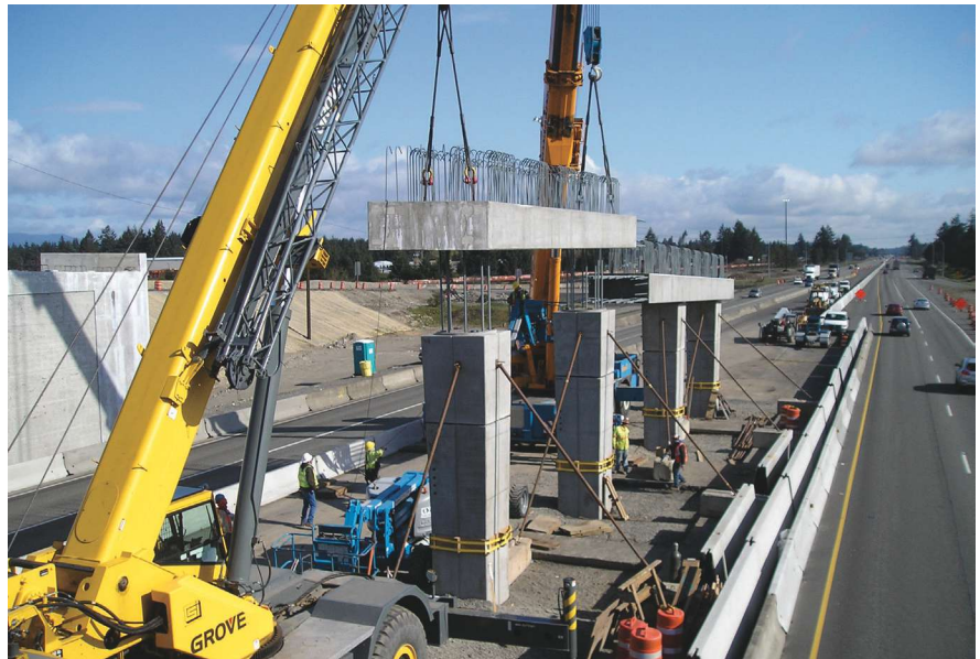
Erection of precast concrete pier cap on precast columns, Interstate 5/US 12 interchange at Grand Mound, Wash. Photo: Patrick Gallagher, Alpha & Omega Group.
