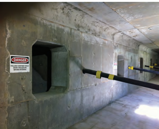
Enclosed outer cells were identified as confined spaces, separately from other interior sections of the bridge segments. Photo: Kenneth Payne.
