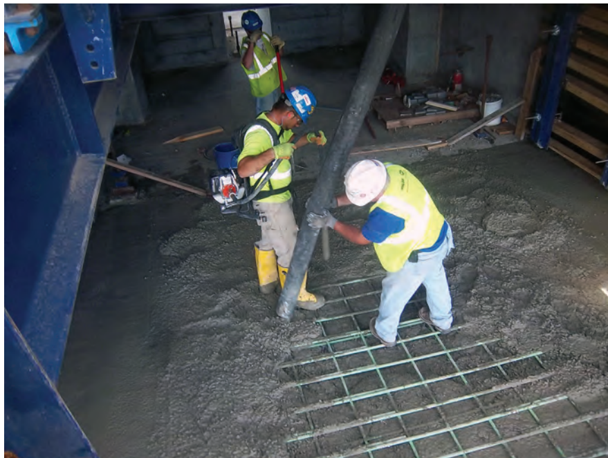
Introduction of a gas-powered concrete vibrator requires a review of the space to determine if it is a confined space. Photo: John Kinkle.
