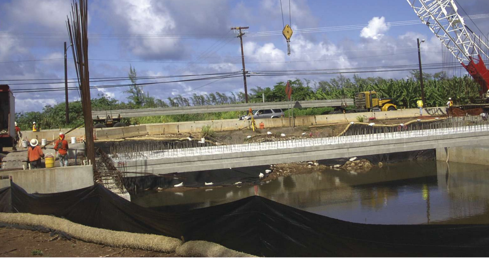
The Kii Bridge, an 80-ft-long, single-span, integral-abutment bridge on Oahu, has a superstructure featuring 2-ft-deep, precast, prestressed concrete planks.
