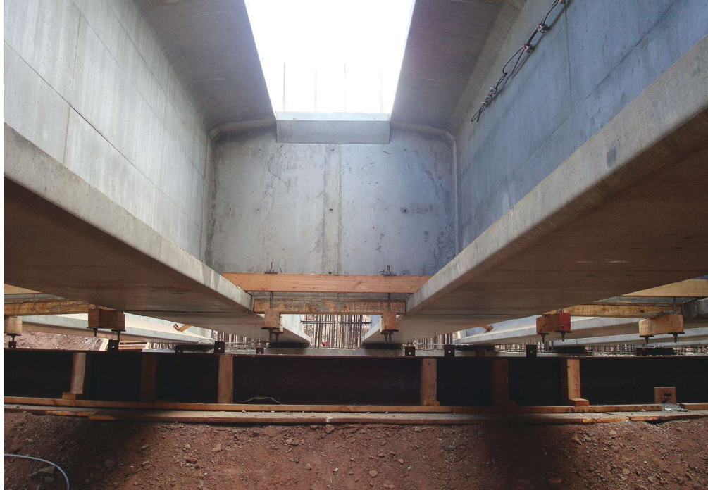
The North-South Road project featured several innovative concepts, including a high-performance concrete deck and a new composition for drilled-shaft concrete. The concrete diaphragm is located at the quarter-point splice between girder segments.
