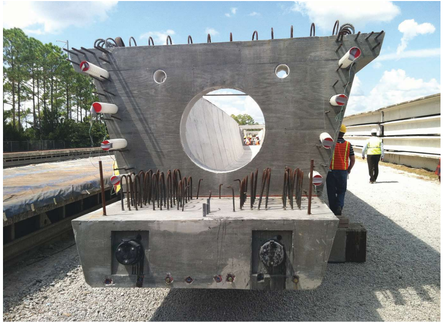
Figure 1. Detail for the expansion end of girder with tongue extension for bearing support. All Photos and Figures: Parsons.
