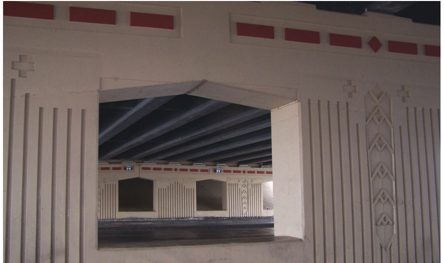
Piers for the new 193 rd Street Bridge in Catoosa, Okla., feature an aesthetic design that was able to meet the requirements of all the stakeholders. Photo: Steven Weitzman/ Creative Design Resolutions.
