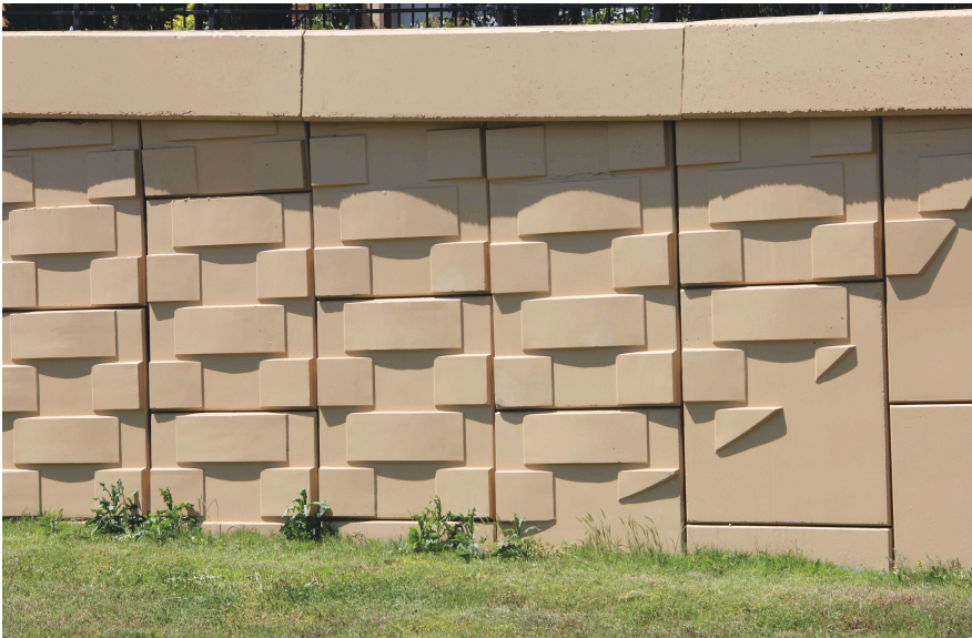
One of the mechanically stabilized earth walls for the 193 rd Street Bridge in Catoosa, Okla., which features an aesthetic design that was able to meet the requirements of all the stakeholders. Photo: Steven Weitzman/Creative Design Resolutions.
