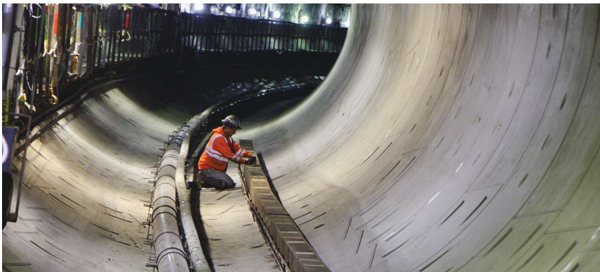
The University Link project is 6 to 9 months ahead of schedule and $150 million under budget. The key challenge was constructing the 23 cross passages between tunnels, which went smoothly.
