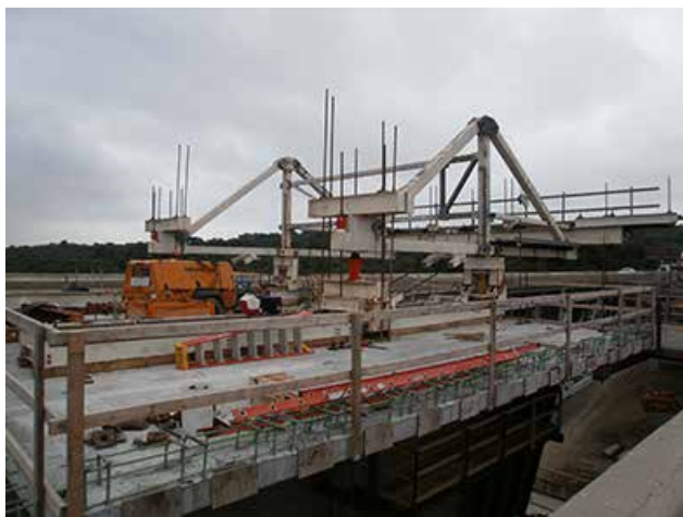
The box girder is cast without the use of scaffolding or falsework using overhead form travelers. Photo: Jeff Weiler, OmniPro Services.
