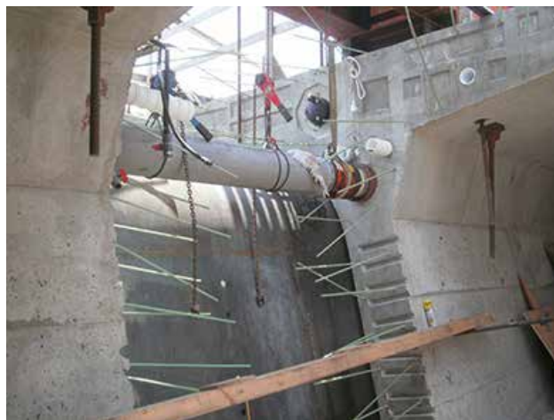
Hydraulic jacks simultaneously pushed grout in-filled steel pipe struts to achieve the specified displacement during the horizontal jacking procedure. The pipe struts were sacrificed within the section, while the jacks were removed following casting of the first-stage 8-ft closure segment. Photo: Jeff Weiler, OmniPro Services.
