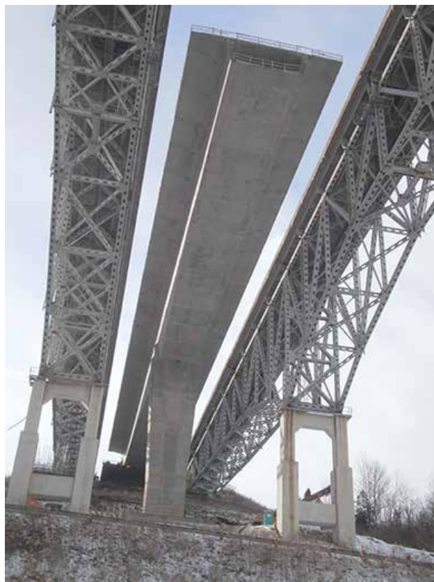
The southbound pier 1 completed cantilever shows the steep terrain conditions necessitating pier column clear heights ranging from 36 to 194 ft. Photo: Jeff Weiler, OmniPro Services.
