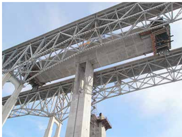
Acting as a fuse element, flexible 65-ft-tall twin-wall piers limit transmitted forces to the substructure below, and are designed to dissipate creep, shrinkage, and thermal effects while providing adequate capacity for external loads. Photo: Jeff Weiler, OmniPro Services.
