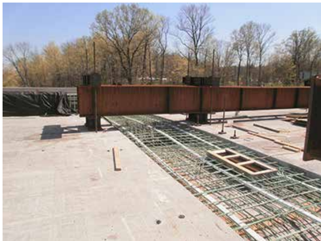
The closure strong-back beams were sized to accommodate forces associated with vertical alignment, and also were required to slide longitudinally during the horizontal jacking procedure while keeping the cantilever tips at the proper elevation. Photo: Jeff Weiler, OmniPro Services.
