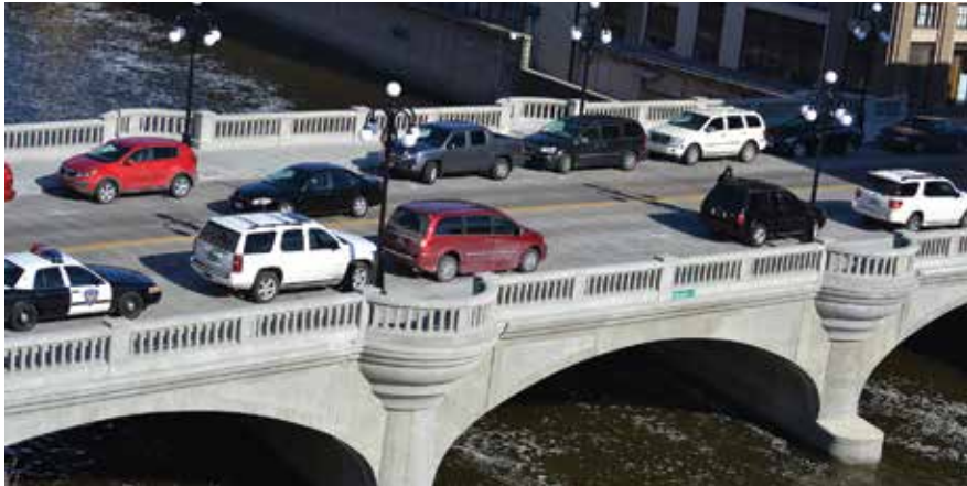
New precast, prestressed concrete deck beam bridge over the East Branch Bridge, as constructed in 2012. All photos: HR Green Inc.
