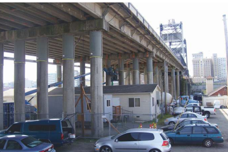
Murray Morgan Bridge port approach with repairs to the tops of the columns in place. All photos: David Evans and Associates Inc.
