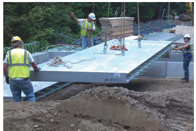
Precast concrete approach slab installation for the State Route 112 Bridge over Kearney Brook. Photo: William E. Dailey Precast LLC.
