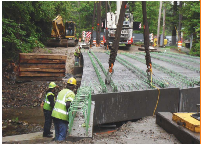
Northeast Extreme Tee (NEXT) beam installation showing the curvature of the flange. Photo: CME Associates Inc.
