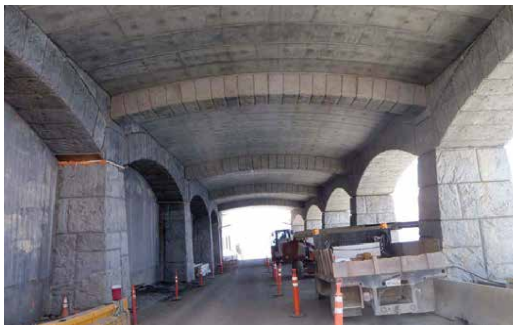
Interior view of the rock shed with roof panels in place, looking south.
