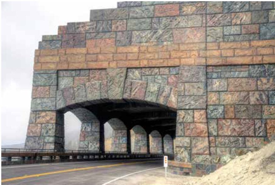
South portal of the Rain Rocks Rock Shed. All photos: California Department of Transportation.
