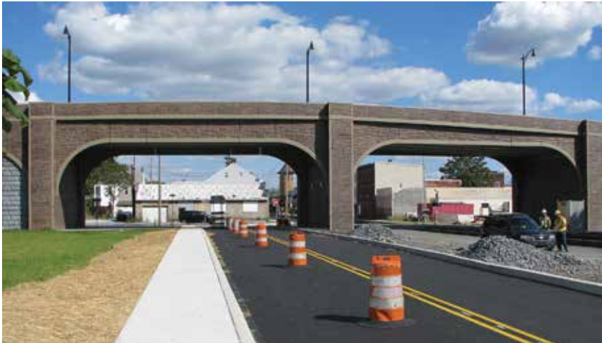
Shown is the 9th Street Bridge overall elevation. Five precast concrete architectural fascia panels per span were suspended from the exterior beams to mimic the look of an historic arch structure. Photo: Troy Jenkins, Northeast Prestressed Products LLC.
