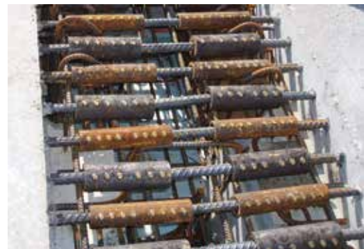
Sibley Pond Bridge showing the use of mechanical couplers. Photo: Parsons Brinckerhoff.
