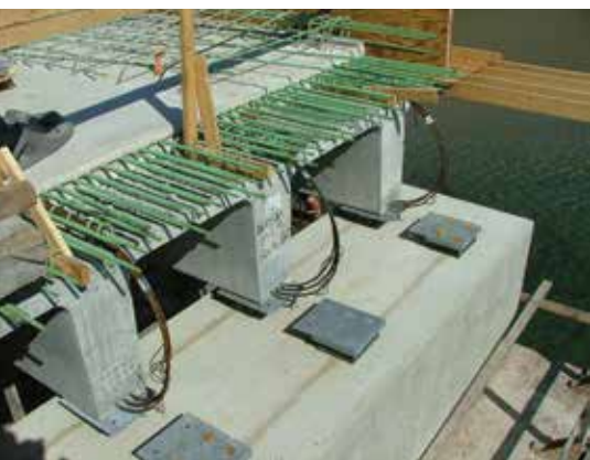
Route 103 Bridge over the York River showing bars extending from the deck. Photo: Vanasse Hangen Brustlin.
