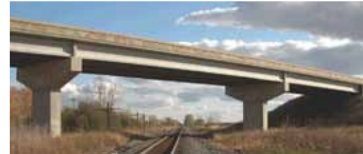
At 377 ft long with four spans, Fond du Lac County's longest bridge carries County Highway RP over the Canadian National Railway.
