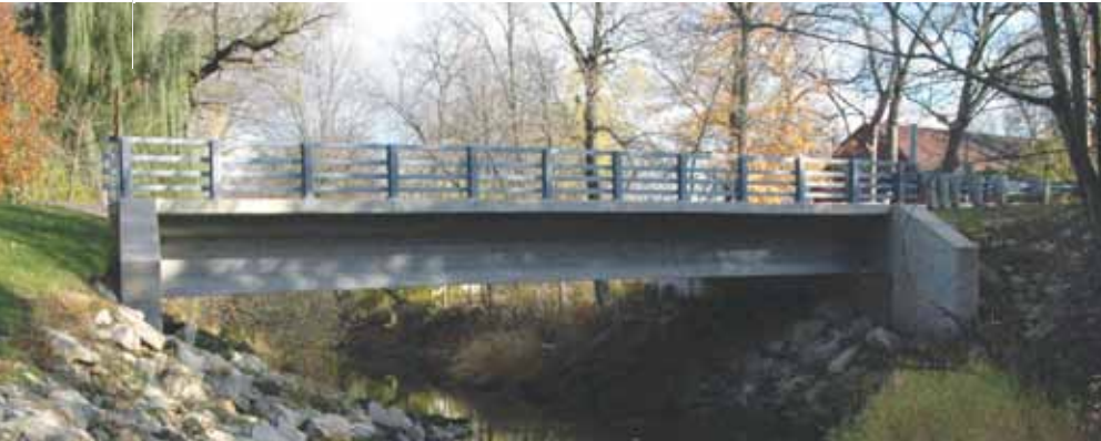
This 65-ft-long span, precast, prestressed concrete girder bridge carries Fond du Lac County Highway C over the West Branch of the Fond du Lac River in Eldorado, Wis.
