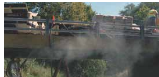
After removing delaminated concrete, sandblasting exposed corroded reinforcement, and painting the reinforcement with an epoxy coating, a Fond du Lac County highway crew applies shotcrete to repair concrete under the deck.
