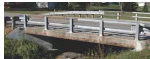
Built in 1921, this concrete slab span bridge carries County Highway Q over the South Branch of the Manitowoc River. It was widened in 1976 and its deck was resurfaced in 2004. Concrete slab span bridges make up many of the county's bridges.
