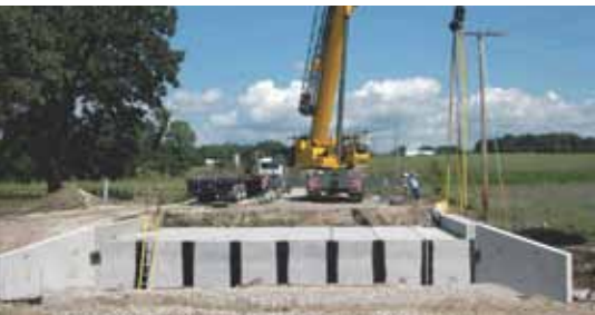
A Fond du Lac County highway crew is shown installing a 20-ft span, three-sided precast concrete structure to carry County Highway B over Parsons Creek.
