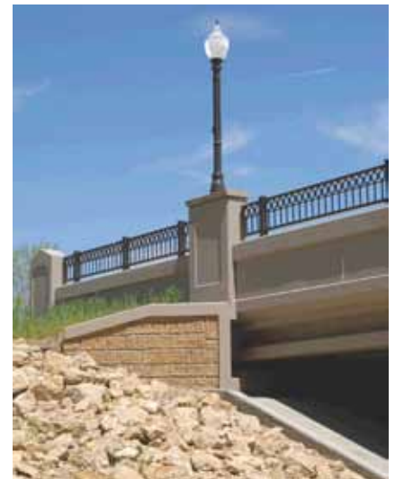
Northwest corner showing aesthetics, including railing post and insets replicating the covered bridge. Photo: MnDOT.
