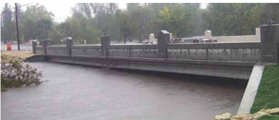
The Zumbro River shown at flood stage on September 23, 2010, toward the conclusion of construction. Photo: City of Zumbrota.
