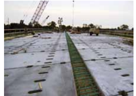
The Parkview Avenue Bridge uses five different types of precast components. Full-depth deck panels are shown after installation before grout placement in the joints and pockets.
