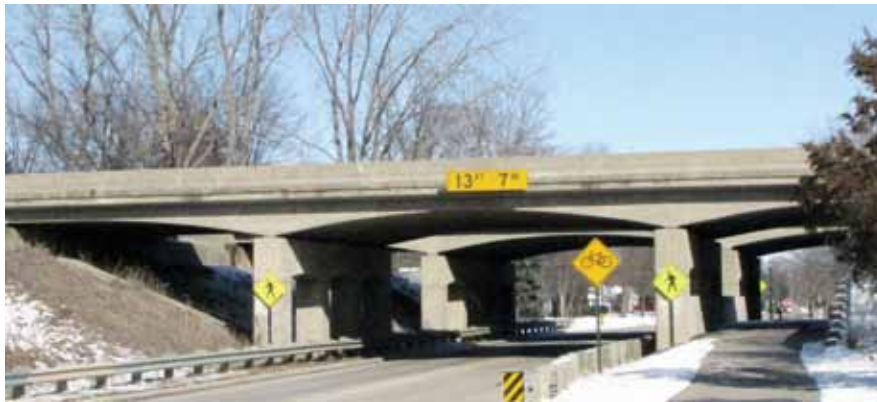
A typical parabolic reinforced concrete T-beam bridge built commonly in the 1950s.
