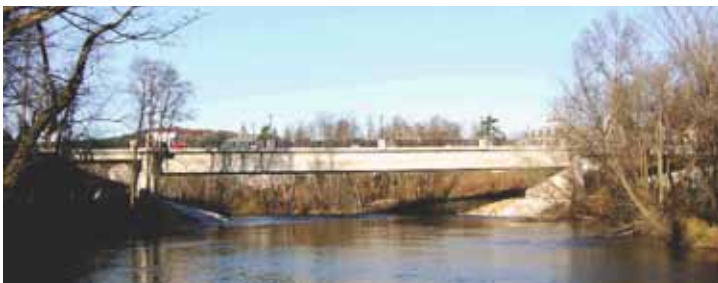
The three-span Cross Street Bridge in Middlebury, Vt., was the first bridge built in the state using the design-build delivery method. Corven provided engineering for the spliced precast concrete girders. Photo: Vanasse Hangen Brustlin Inc.
