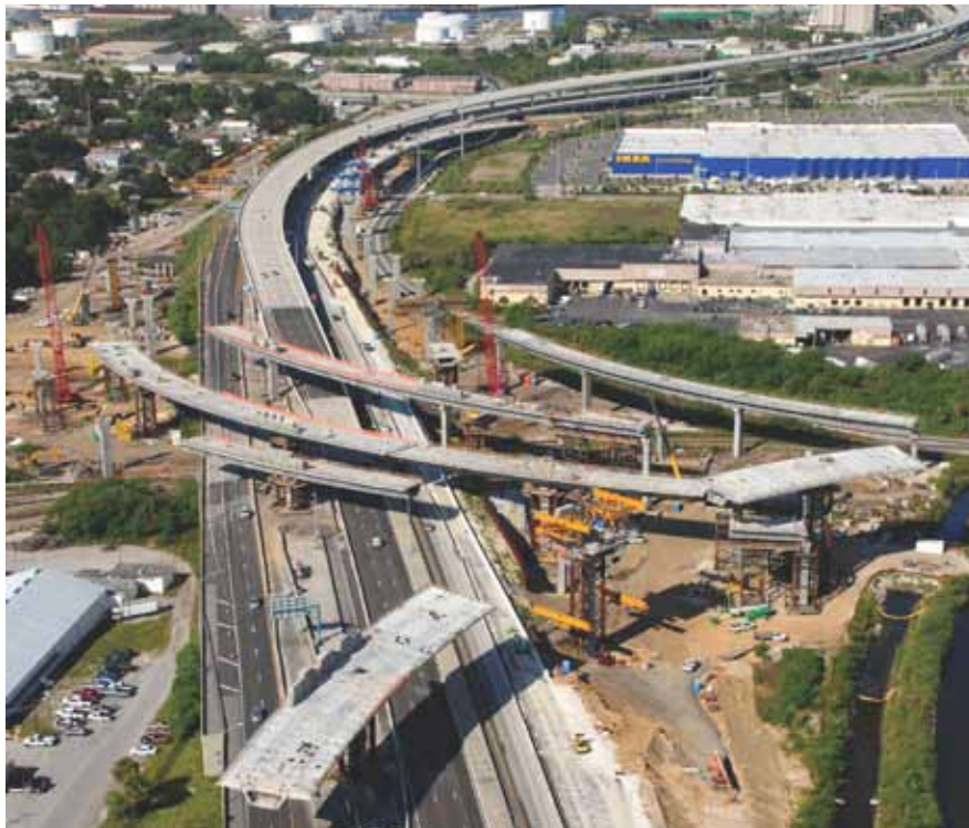
On the I-4/Lee Roy Selmon Expressway Interchange in Tampa, Fla., Corven is providing construction engineering services to a joint venture of PCL Civil Constructors and Archer Western Construction. The project includes more than 2500 precast segments that vary in width from 30 to 60 ft. Photo: PCL Civil Constructors and Archer Western Construction, joint venture.
