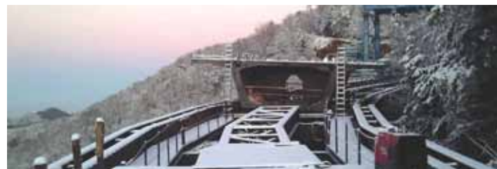
The 790-ft-long Foothills Parkway Bridge No. 2 near Wears Valley, Tenn., is a precast segmental concrete bridge with span lengths up to 180 ft. Corven supplied design and construction engineering services to Bell & Associates Construction. Photo: Corven Engineering Inc.
