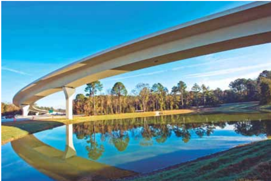
The balanced-cantilever method was used to construct the I-95/I-295 North Interchange Ramp in Jacksonville, Fla., for which Corven provided construction engineering services. The bridge features precast concrete segmental box girders in a 10-span continuous configuration with a total length of 2256 ft. Photo: Superior Construction Company.
