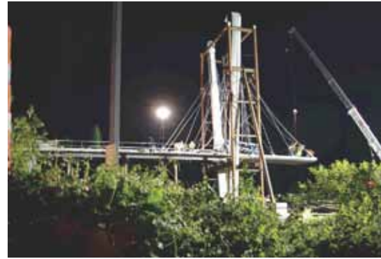
Daytime closures on Delta Highway were out of the question, so crews erected the precast concrete pylon tower and placed the precast deck panels at night.
