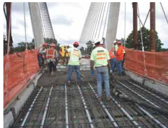
Placing the main span topping slab on the precast panels. The longitudinal post-tensioning ducts can be seen between the curbs of the precast panels.
