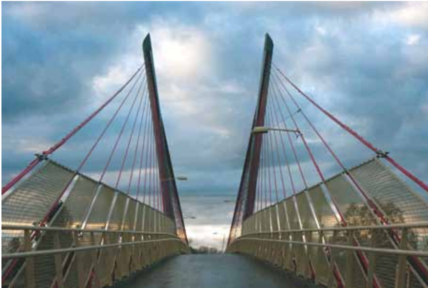
The structure's concrete V-shaped pylon tower is an impressive sight for bikers and pedestrians as they cross the Delta Ponds Pedestrian Bridge.
