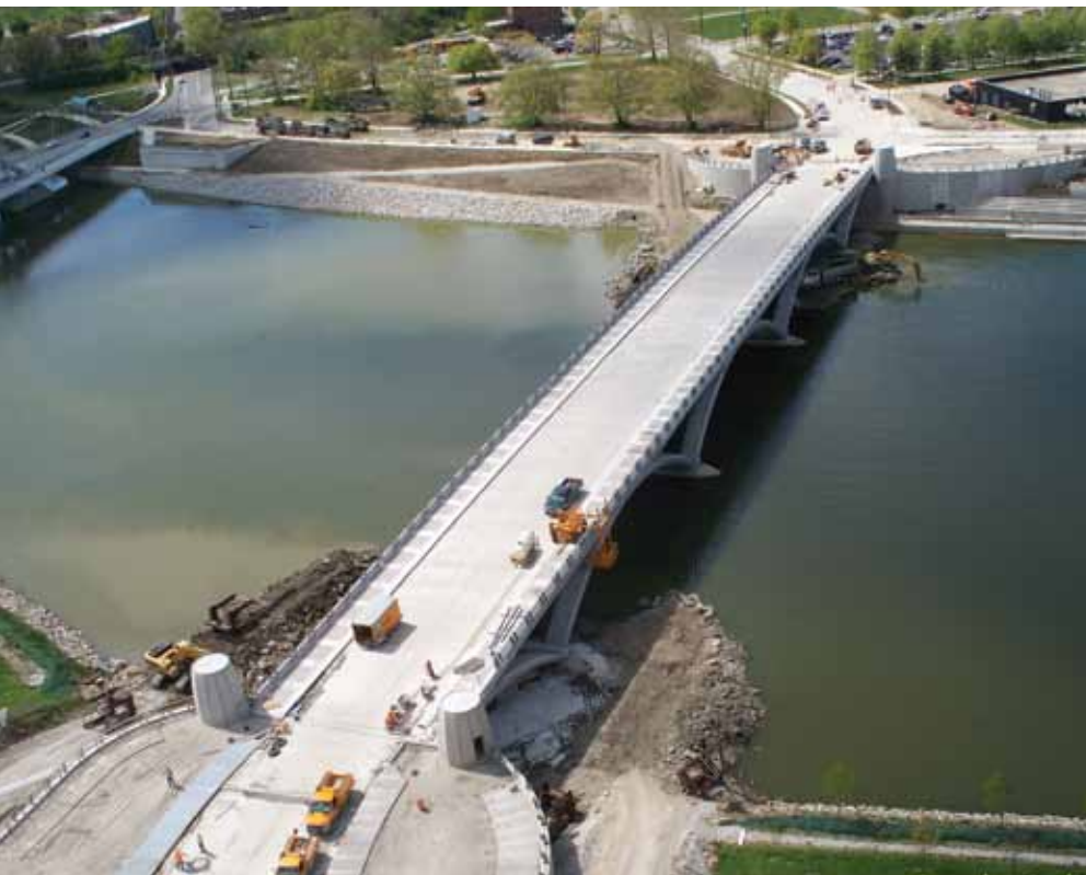
Aerial photograph after the bridge deck was placed. Photo: Ohio Department of Transportation District 6.
