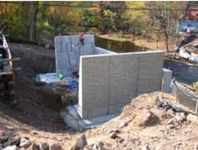
The wingwalls were 22 ft tall and tapered in thickness from 3 ft 10 in. to 1 ft 6 in. Photo: Arborio Corporation.
