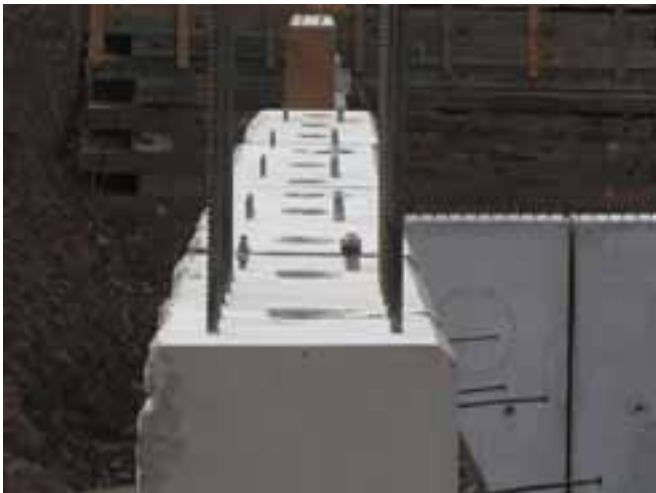
The top edges of the wingwalls had provisions to mount the rail posts and attach the cast-in-place concrete end block. Photo: Hoyle, Tanner & Associates Inc.
