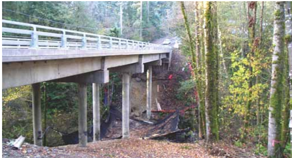
The Wynaco Bridge spanning Covington Creek was extensively rehabilitated to upgrade its load capacity, seismically retrofit it, and strengthen its rails. The 195-ft-long bridge reused some precast concrete girders with a more efficient spacing, saving time and money. The project won two awards from the local American Society of Civil Engineers.
