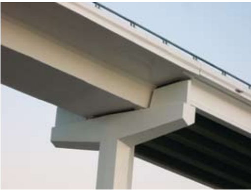
The transition pier showing the ear walls to hide the ends of the precast, prestressed concrete beams. Photo: Dean Van Landuyt, TxDOT.
