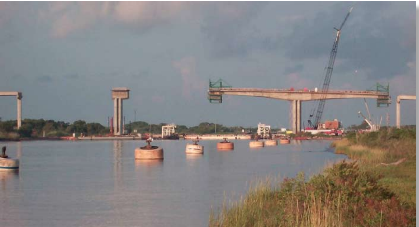
The state of segmental construction just 2 weeks prior to the arrival of Hurricane Ike. Photo: Keith Kouba, TxDOT.
