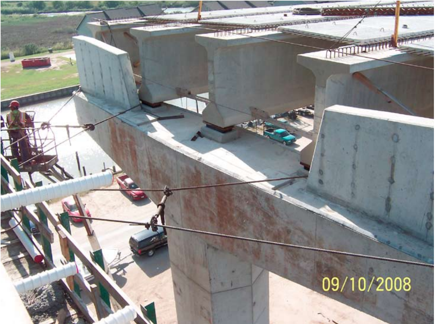
Temporary cables were secured to the ear walls of the transition piers to reduce column torsion expected from Hurricane Ike. Photo: Keith Kouba, TxDOT.
