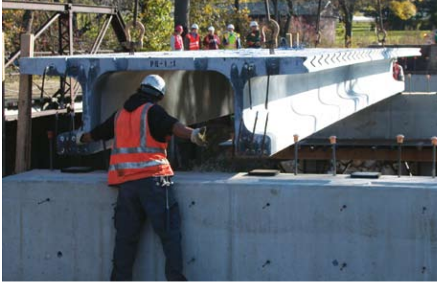
The 50-ft simple-span Pi girders are supported on plain neoprene bearing pads.
