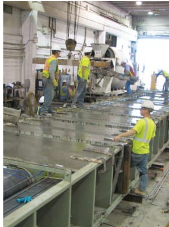
The precaster cast two 25-ft-long beams for testing purposes by the FHWA, followed by three 51-ft-long production beams.
