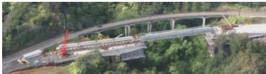
The center span is shown under construction. One girder has been launched and a second is being assembled in the staging area.
