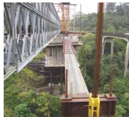
After each girder was lifted, the launching truss was moved laterally and the girder set in its final position. Photo: Eric Y. Matsumoto, KSF Inc.
