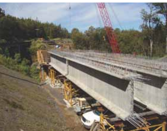
Two precast girder segments, 50 ft long, were set on falsework and spliced together for the end spans. Photo: Eric Y. Matsumoto, KSF Inc.
