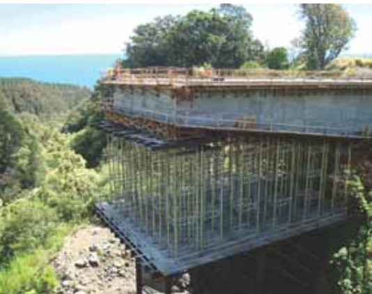
The 150-ft-long, cast-in-place concrete box girder above Pier 2 was cast on falsework and post-tensioned prior to launching the spliced girder drop-in span. Photo: Eric Y. Matsumoto, KSF Inc.
