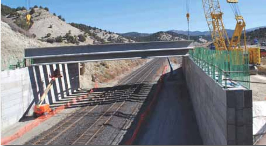
The Mile Post 200 Bridge provides a new alignment of U.S. 6 over UPRR tracks. Type VI AASHTO girders bear on an abutment framed with precast concrete blocks stacked 33 ft high. The blocks are keyed and post-tensioned to the footing. Photo: Utah Department of Transportation.
