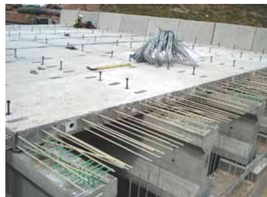
This end panel with integral barrier will connect with the cast-in-place concrete end closure diaphragm. The panels are also connected together with a cast-in-place longitudinal closure strip along the center of the bridge. Photo: Utah Department of Transportation.
