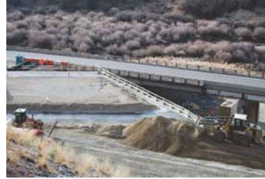
The old Mile Post 200 Bridge is seen in the background. The new alignment will have U.S. 6 traverse a reverse curve diagonally across the new bridge in the foreground. The new concrete girders span nearly up and down in the photo. Granular fill is being placed on the structure to create the reverse superelevation of the new alignment. The roadway will be paved with asphalt. Photo: Utah Department of Transportation.
