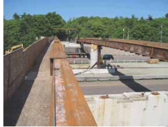
The original steel bridge's I-girders were removed and then reused as temporary erection beams to support the precast concrete channel segments during erection. Photo: Purcell Associates.
