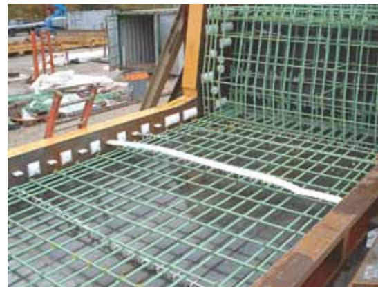
The precaster purchased relatively simple specialized forms to cast the channel segments shown here during set-up for casting the first non-match-cast segment. Photo: IBT.
