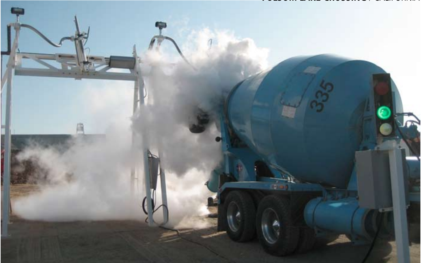
Kiewit constructed a liquid nitrogen plant to lower the initial temperatures of the concrete for mass concrete placements.
