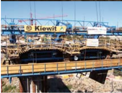
Form traveler for cast-in-place segmental construction advancing from the pier table. Portions of the travelers were last used on the nearby Benicia-Martinez Bridge project.
