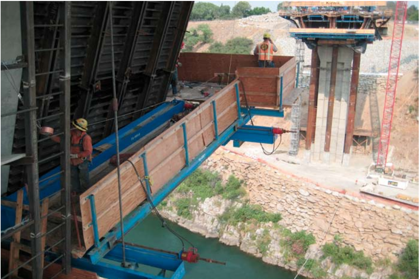
Looking from the Pier 3 cantilever towards Pier 2, shows the height of the structure over the water and the reconstruction efforts required for the slope
