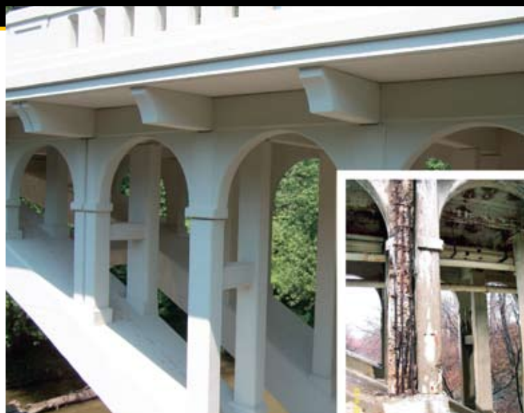
Precast concrete components, including columns and spandrel walls were carefully fabricated to replicate the look of the original concrete pieces replaced on the historic Spring Street Bridge in Floyd and Clark Counties, Ind.
