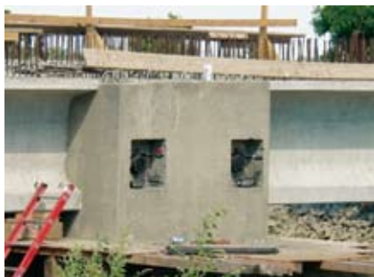
The integral post-tensioned bent caps transferred longitudinal moment between the columns and the superstructure. Photo: Con-Fab.
