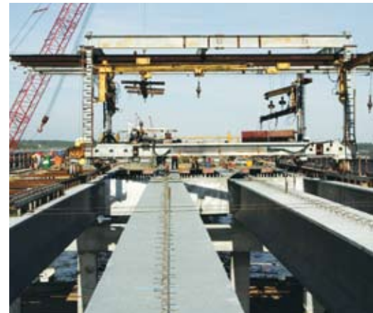
A track-driven placer was used to install the steel formwork for the deck.
