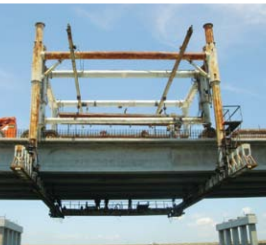
A deck stripper was used to remove the steel formwork from the underside of the deck.
