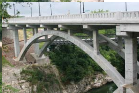
The new Lime Kiln Bridge replicates the look of the original bridge, which was one of the first open-spandrel, concrete arch bridges in the United States and the first in Vermont.
