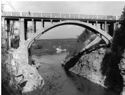
The original bridge built in 1913 was substantially rehabilitated in 1940 shown here and 1991.
