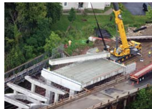
The end spans feature precast, prestressed concrete butted box beams that were transversely post-tensioned after placement.
